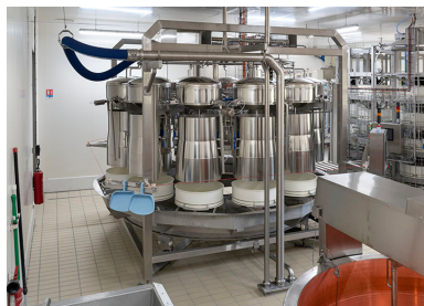
Installation de moulage. Phot. Sonia Dourlot IVR43_20192500951NUC4A
