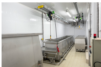
Bain de saumure. Phot. Sonia Dourlot IVR43_20182501705NUC4A
