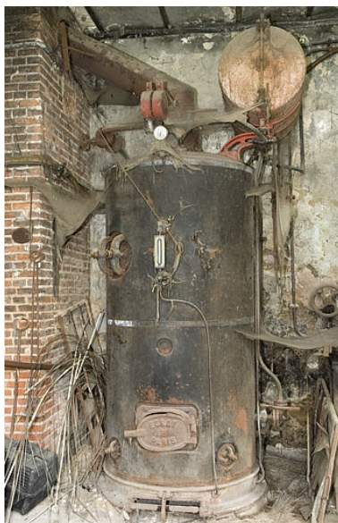
Atelier de distillation. Chaudière Egrot. Phot. Jérôme Mongreville IVR43_20067000677NUCA
