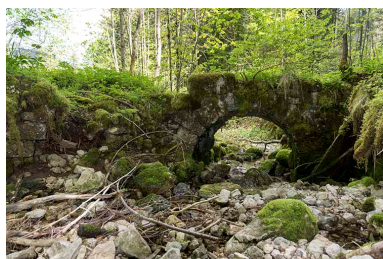
Pont en ruine. Phot. Sonia Dourlot IVR43_20172500614NUC4A
