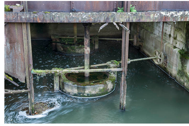
Turbines Douge. Phot. Jérôme Mongreville IVR43_20142501648NUC4A
