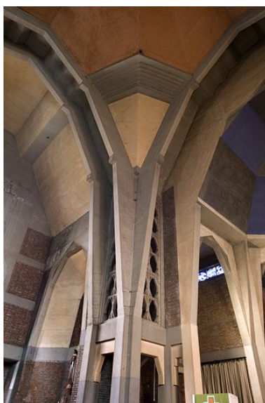
Pilier. Phot. Yves Sancey IVR43_20062500704NUCA
