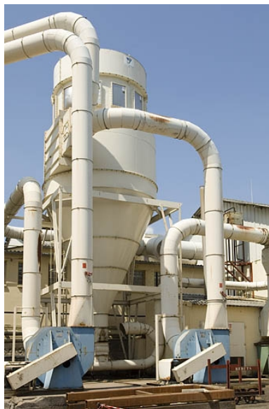
Silo de sciure. Phot. Jérôme Mongreville IVR43_20097000753NUC2A
