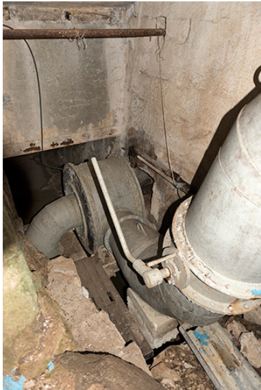
Turbine. Phot. Sonia Dourlot IVR43_20172501778NUC4A
