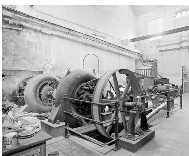
Turbine Francis (1929). Phot. Yves Sancey IVR43_19999000288X
